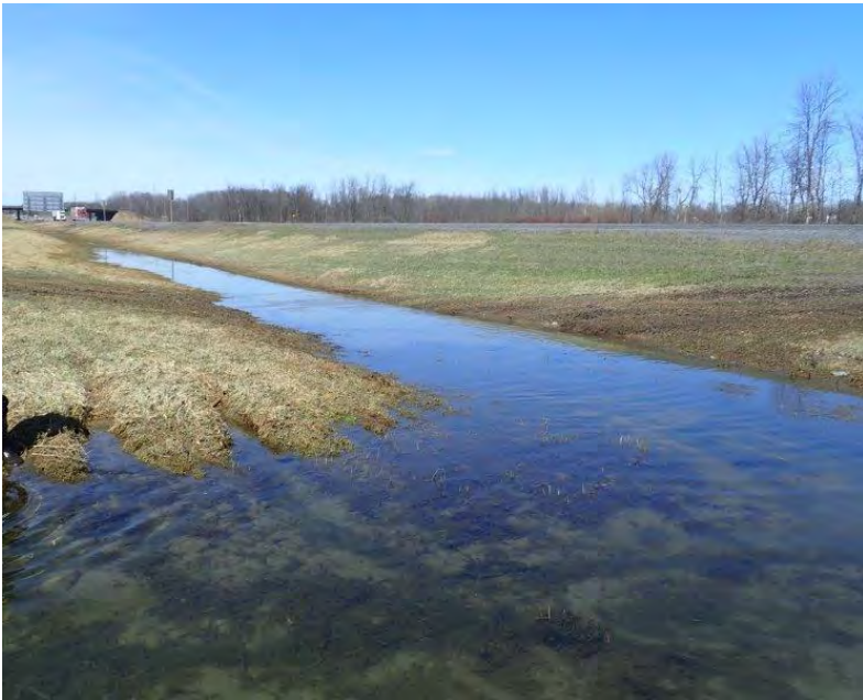
Photo 31. C22 – Highway 401 – View of the inundated ditch line and standing water near culvert outlet. April 11, 2022
