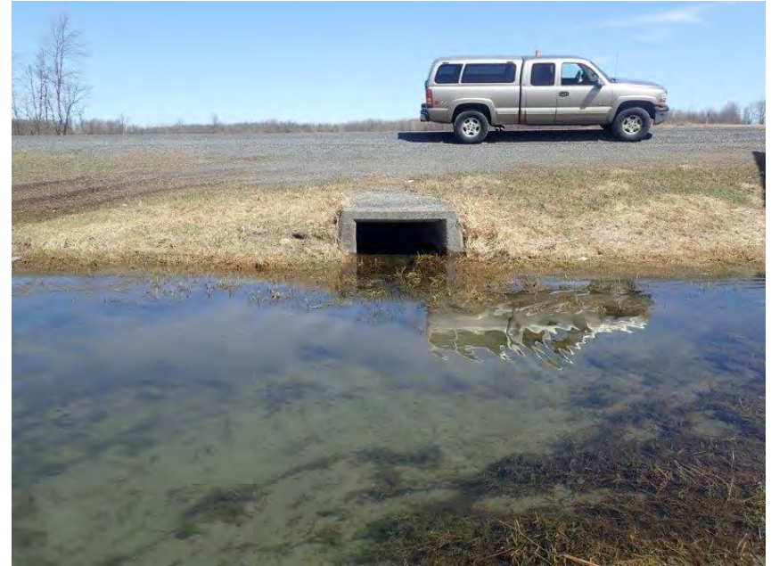
Photo 30. C22 – Highway 401 – View of the outlet with standing water. April 11, 2022
