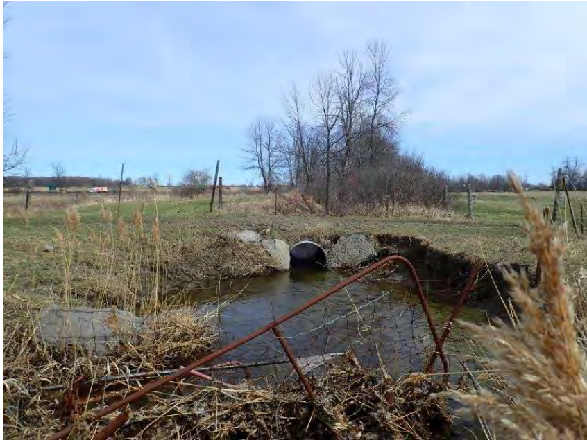
Photo 17. C17 – Power Dam Drive – View of the downstream channel and downstream secondary culvert. April 11, 2022
