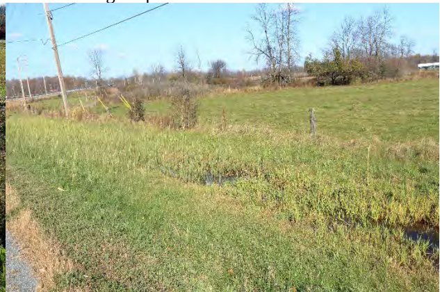
Image 48: North view along the east side of Power Dam Drive showing deep ditch.
