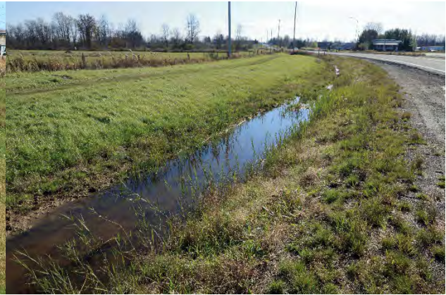
Image 44: South view along the east side of bridge approach of Power Dam Drive showing deep ditch.
