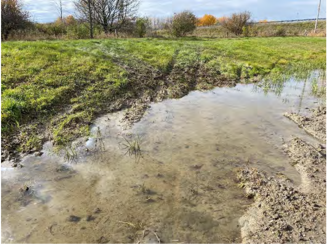
Figure 45: South side of Hwy 401, ditches compromised by ATV tracks causing interference with drainage
