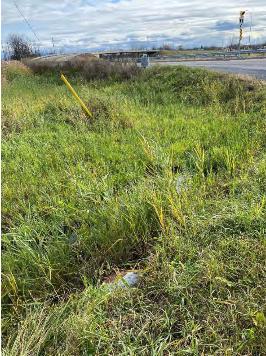
Figure 47: C4 - Culvert under Power Dam Drive on North side of Hwy 401, with ponding
