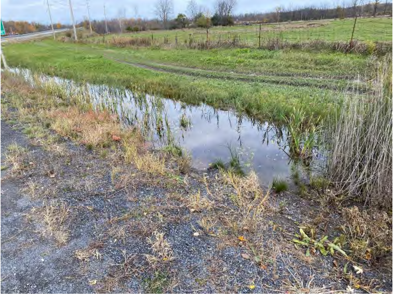
Figure 9: Ponding along Power Dam Drive caused by tire tracks from Figure 7, 8
