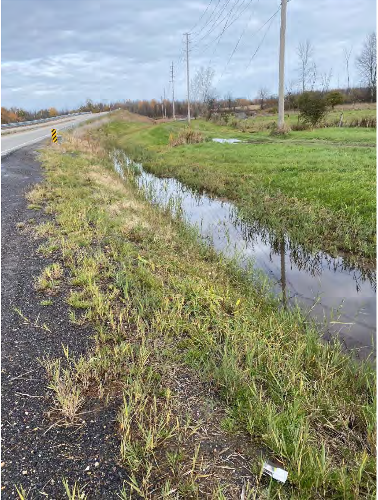
Figure 10: Ponding along Power Dam Drive caused by tire tracks from Figure 7, 8
