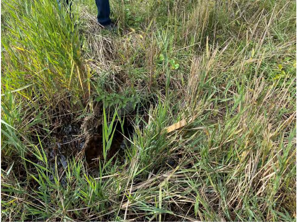
Figure 19: C8 outlet, rusted, mostly embedded, poor flow
