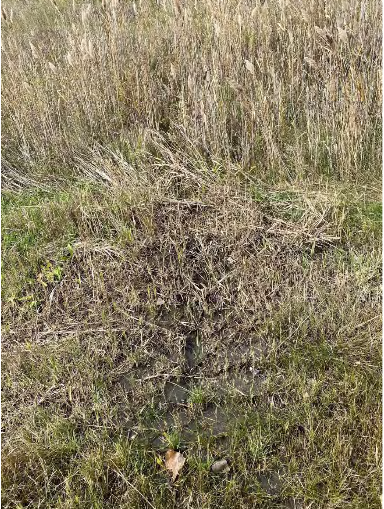
Figure 15: Seepage from CB outlet (SSC9/C13)
