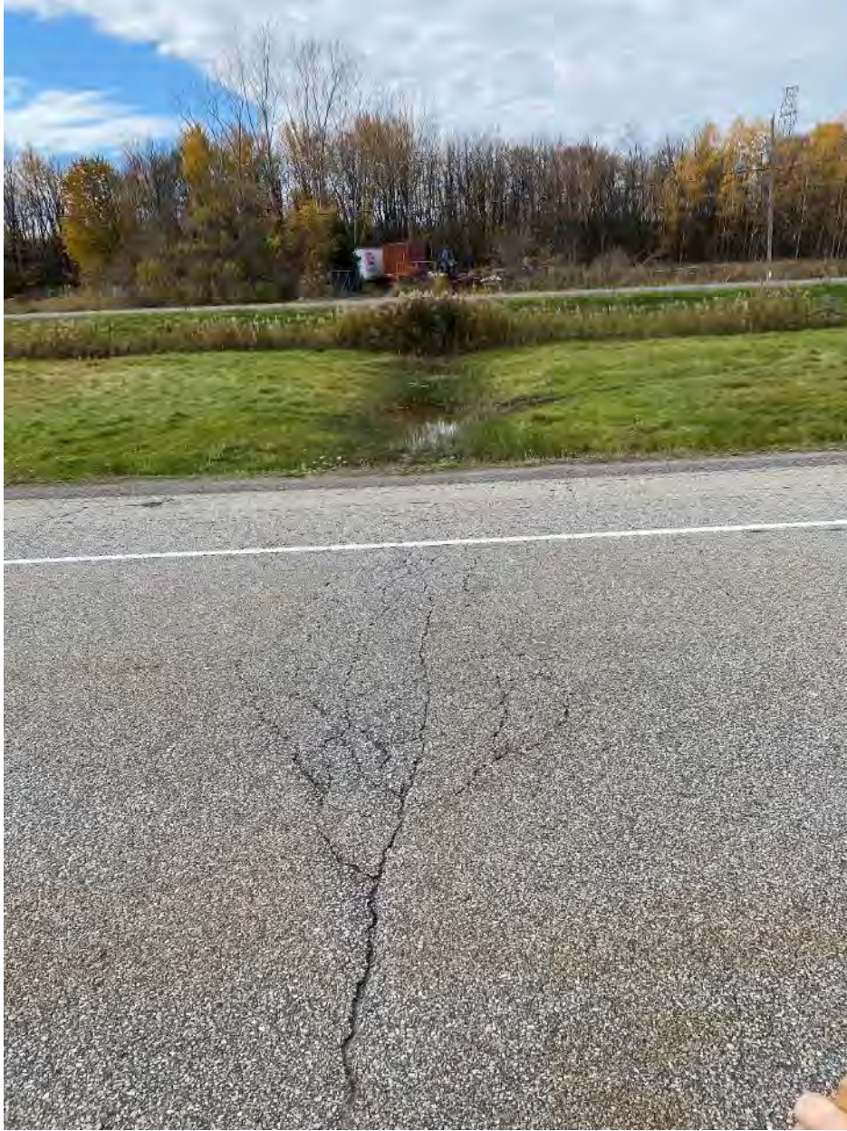
Figure 30: Road surface wear and upstream ponding of Culvert C7 (Hwy 401 offramp)
