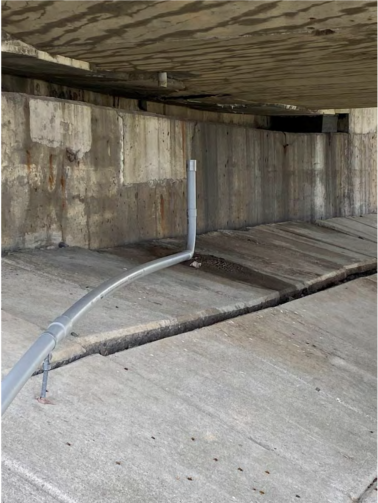
Figure 21: Disconnected Deck Drain outlet S-E side of Power Dam Drive
