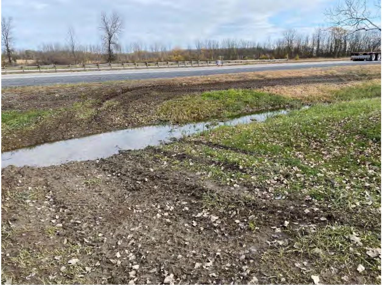
Figure 17: Ponding on DS side of C8, ruts caused by ATV limit drainage
