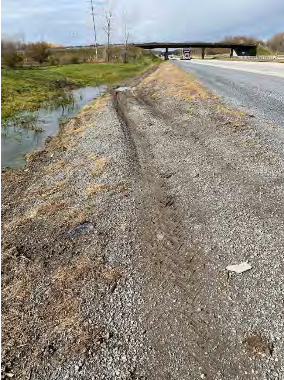
Figure 44: South side of Hwy 401, ditches compromised by ATV tracks causing interference with drainage
