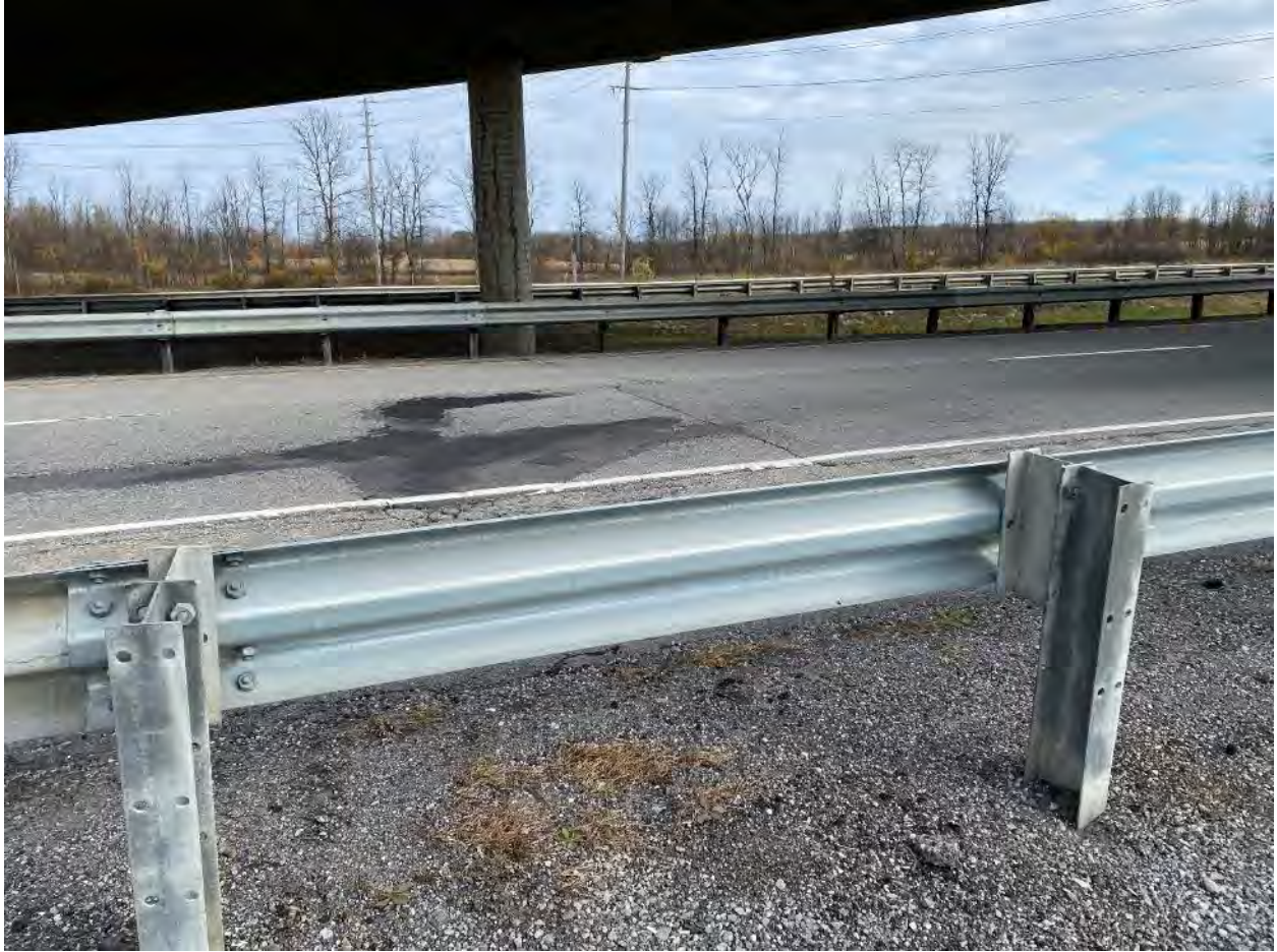
Figure 24: Damage to Hwy 401 EB under Power Dam Drive
