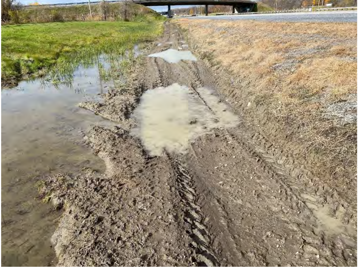
Figure 46: South side of Hwy 401, ditches compromised by ATV tracks causing interference with drainage
