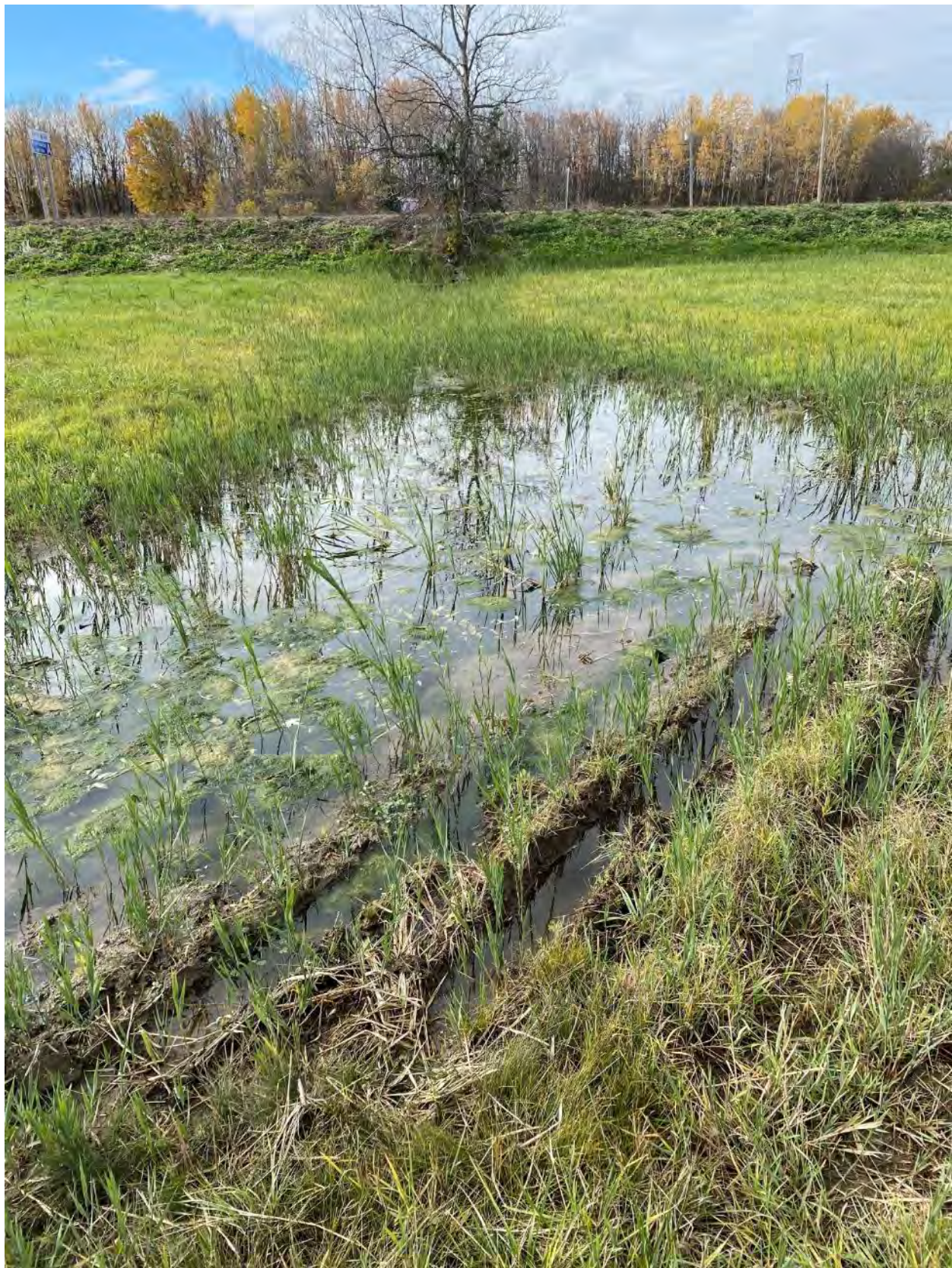
Figure 25: Ponding at DS outlet of C5 and confluence of C7 South of Hwy 401
