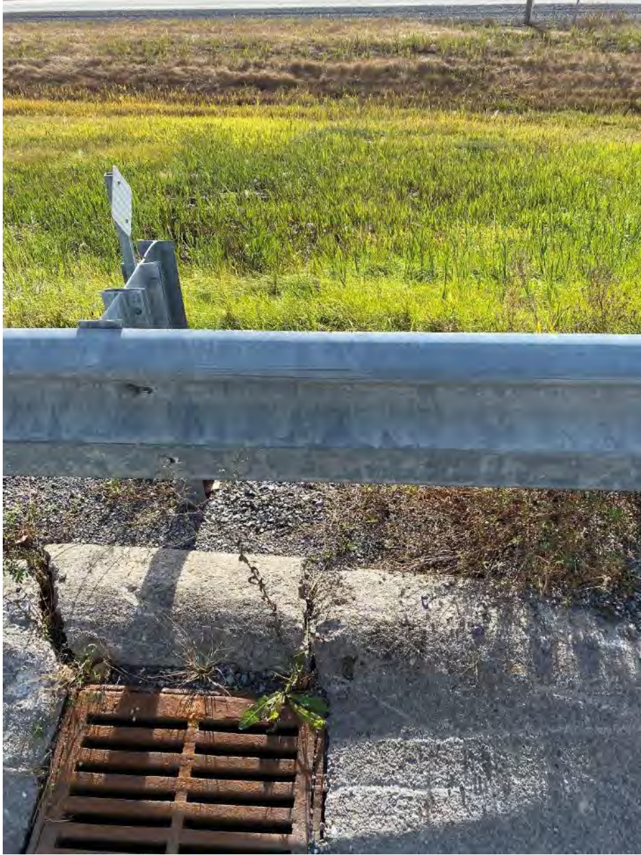
Figure 52: CB and SSC7, with wet area below. No outlet could be observed.
