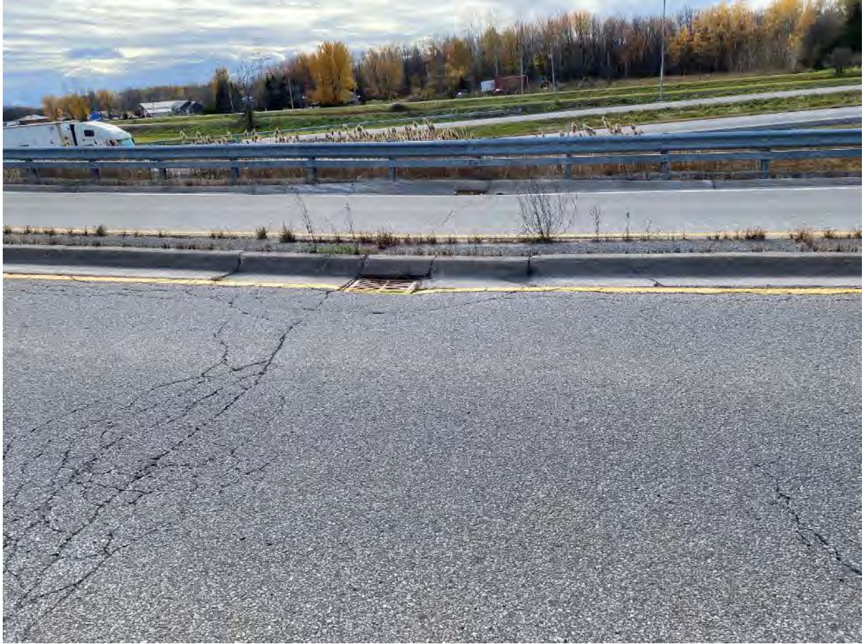
Figure 50: SSC8, CB (x2) and lead to south side of Power Dam Drive
