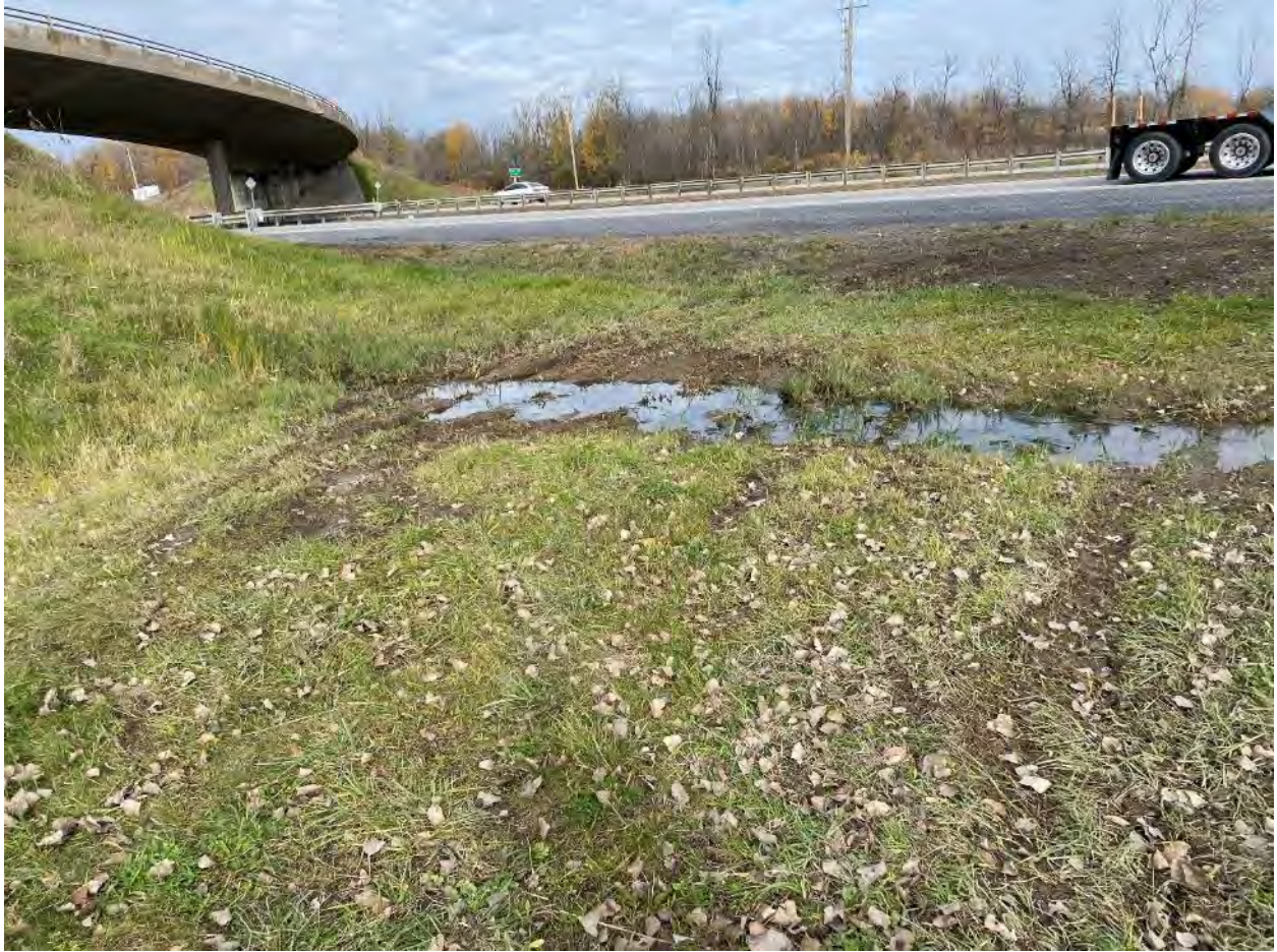
Figure 16: Ponding on DS side of C8, ruts caused by ATV limit drainage
