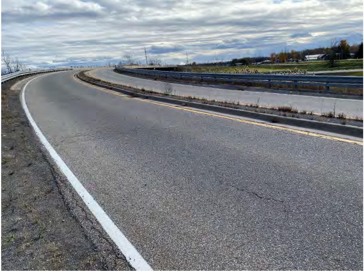
Figure 49: SSC8, CB (x2) and lead to south side of Power Dam Drive
