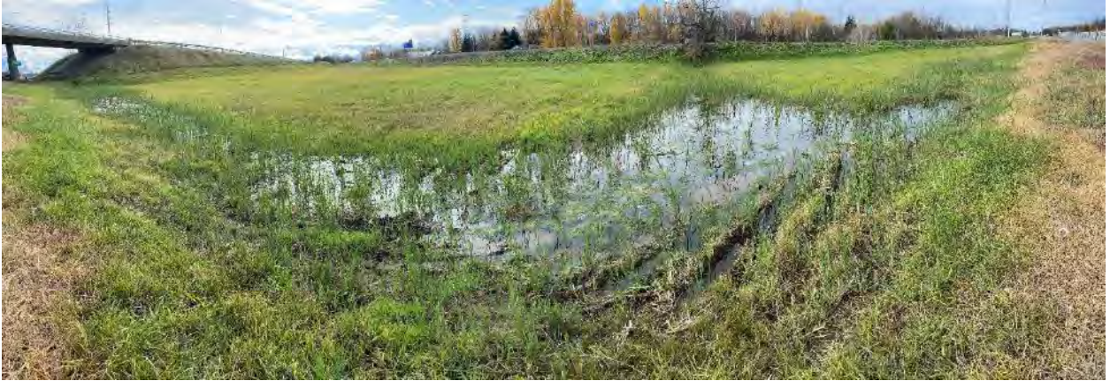
Figure 26: Ponding in area between Hwy 401, Hwy 401 off-ramp and Power Dam Dr.
