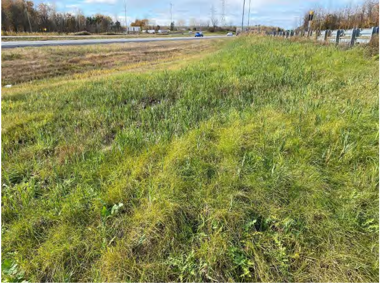
Figure 51: Outlet area of SSC7; no outlet could be located, but wet soil conditions encountered.
