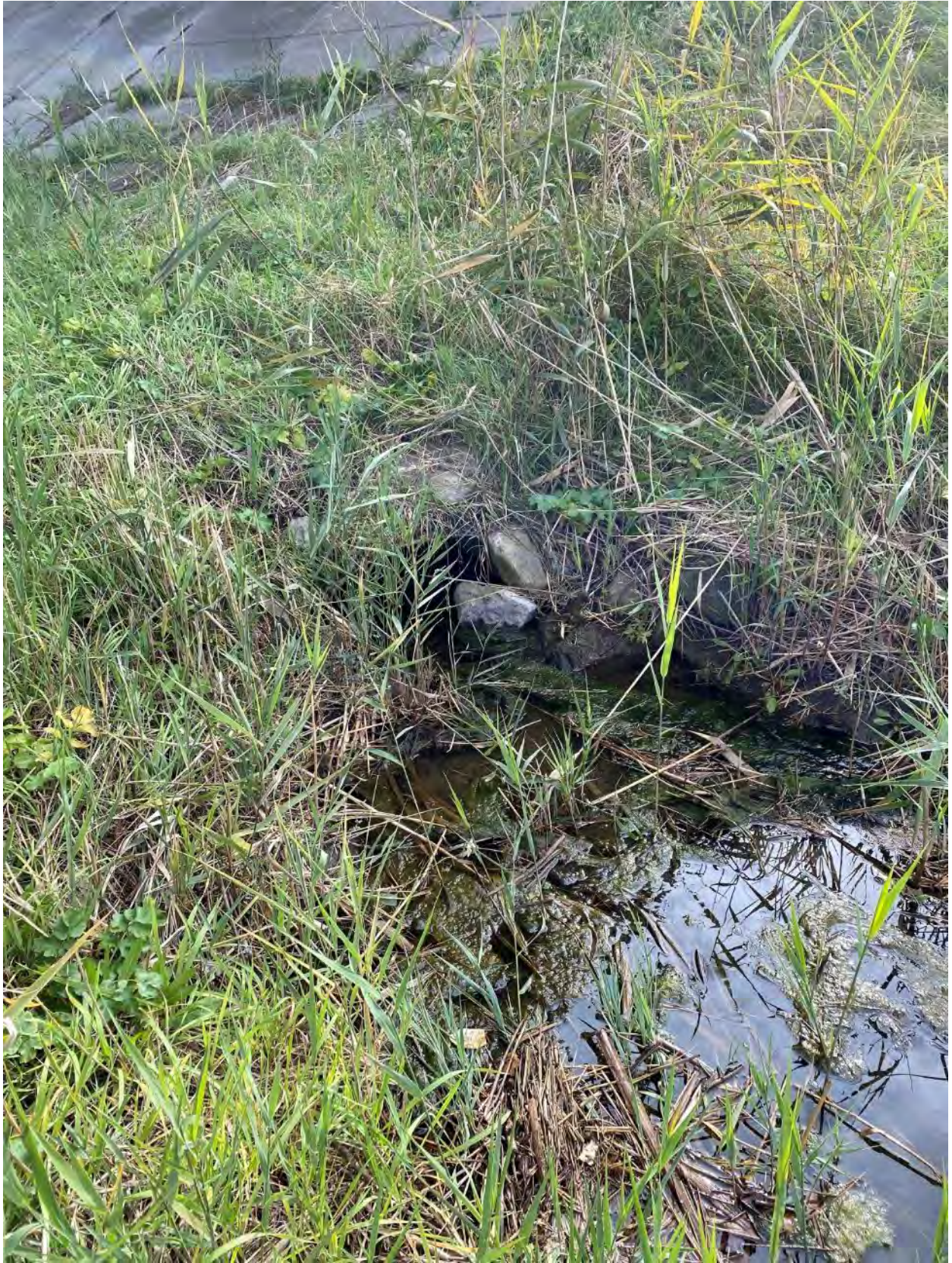
Figure 22: Inlet of C8, partially blocked, ponding observed
