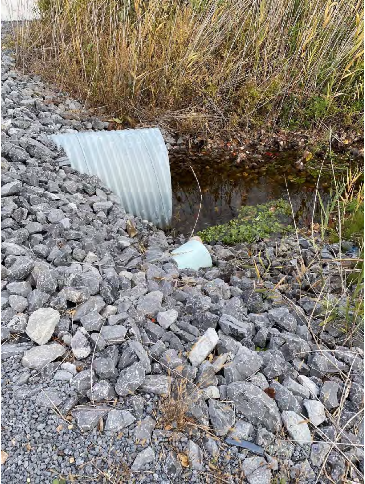
Figure 6: Outlet of C17 and CB lead at Atchinson Road
