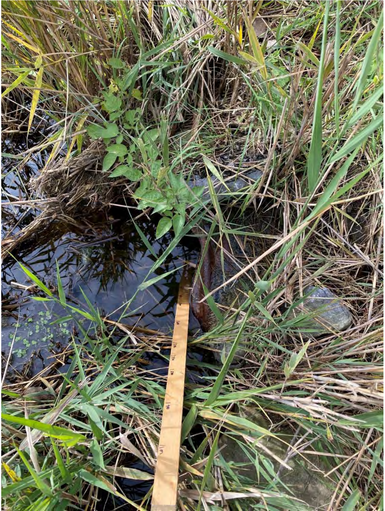
Figure 18: C8 outlet, rusted, mostly embedded, poor flow
