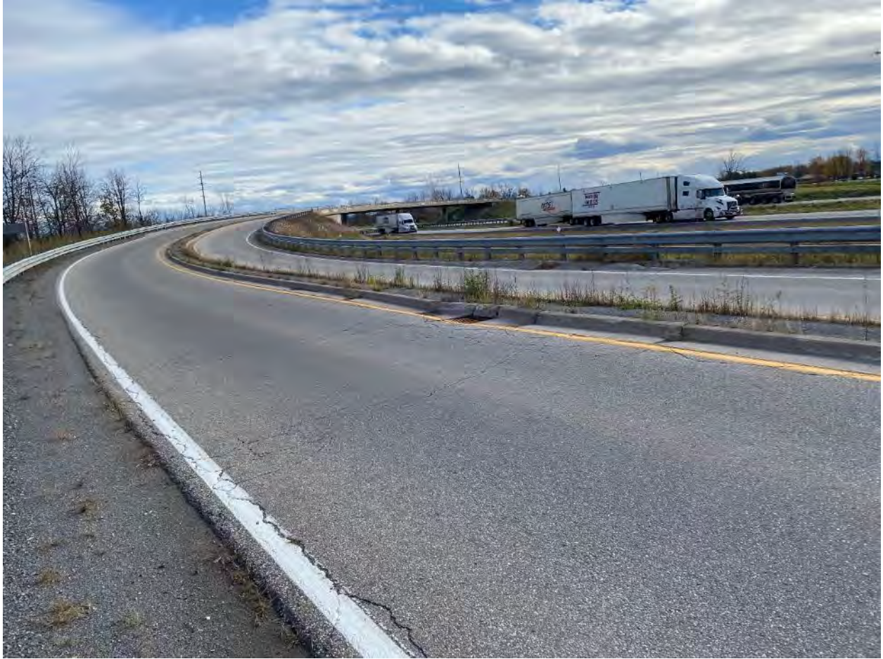
Figure 48: SSC7 - CB (x2) and lead to South side of Power Dam Drive
