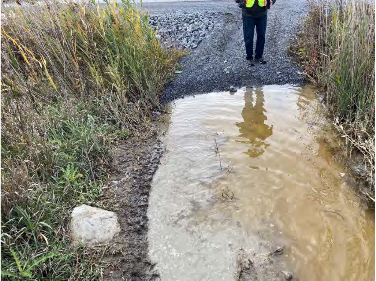
Figure 8: Damage to Drainage Ditch. Ponding caused by tire tracks from ATV
