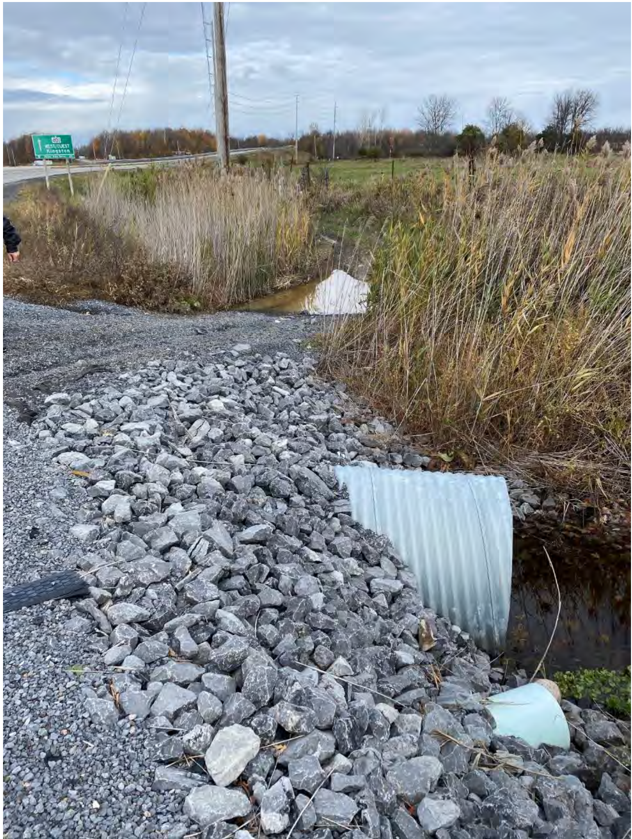
Figure 7: Damage to drainage ditch near outlet of C17
